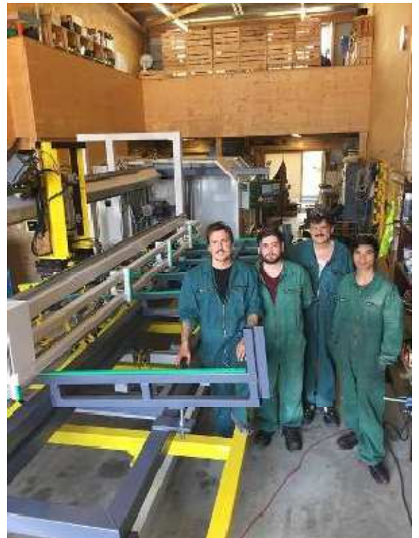
Picture 103: Photo with the installation team from the side of the machine
