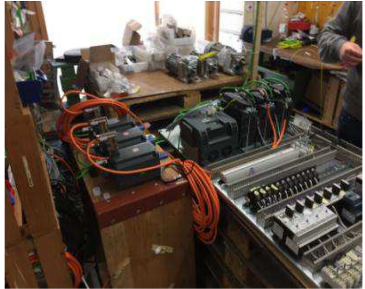
Picture 6: Everything is set up for testing, so that when we have the machine mechanically finished, everything has been running and is preset
