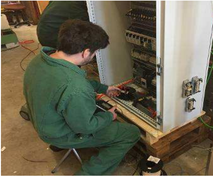
Picture 57: Sven at E cabinet assembly
