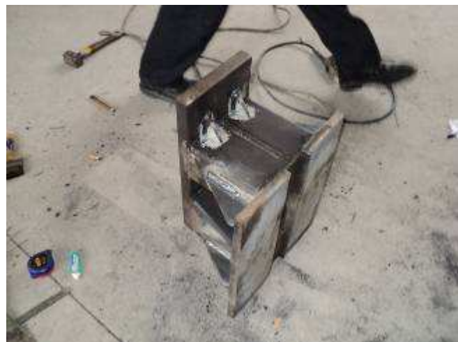
Photo 15: Now Robinson has the tailstock bracket welded ready yet, so he makes a lot. We must be careful that the teachers do not always catch only the most beautiful work. The teacher then left the apprentices not so nice work.
